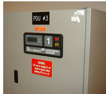
Figure 9. Power Distribution Unit (PDU) near Row F.
