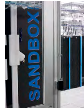
HP's Fort Collins Research Lab datacenter
